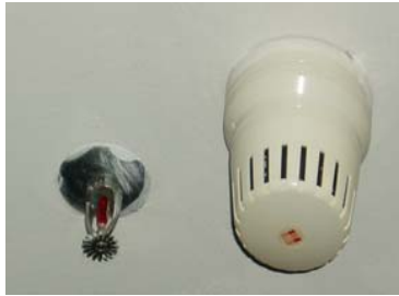
Gambar 4. Sprinkler & Smoke detector
